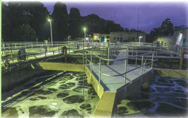
NIGHTWATCH AT THE PLANT in adherence with COVID-19 guidelines, CAWD staff are split into day and night shifts to ensure that we have skilled plant operators even if one shift has to quarantine.
