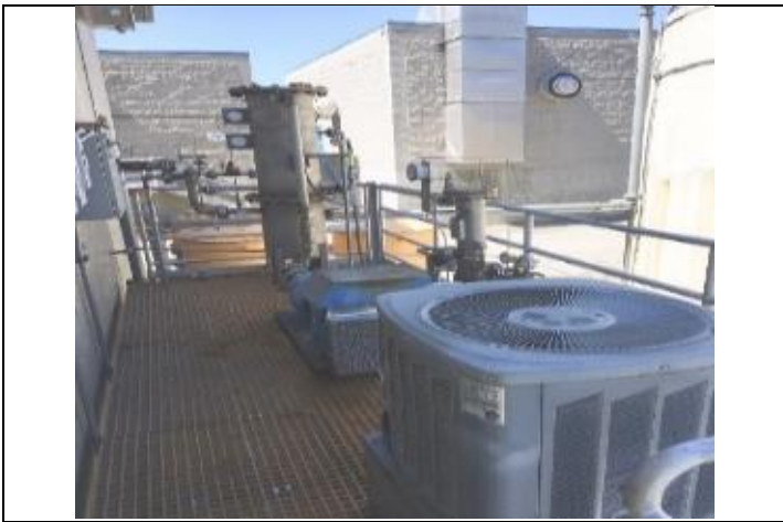
Photo: Existing Gas Conditioning System
