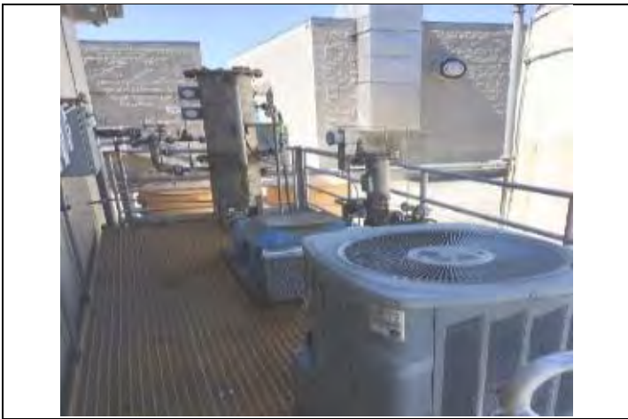
Photo: Existing Gas Conditioning System
