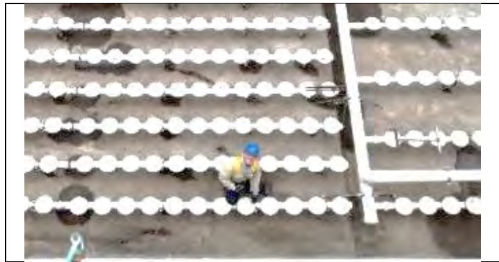
Photo: Existing air diffuser system
