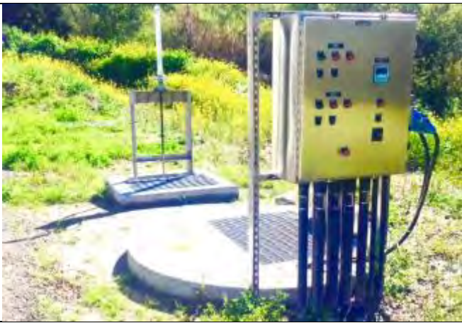
Photo: WWTP Stormwater Pump Station
