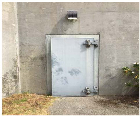
Photo: Old Flood Door in Headworks Basement
