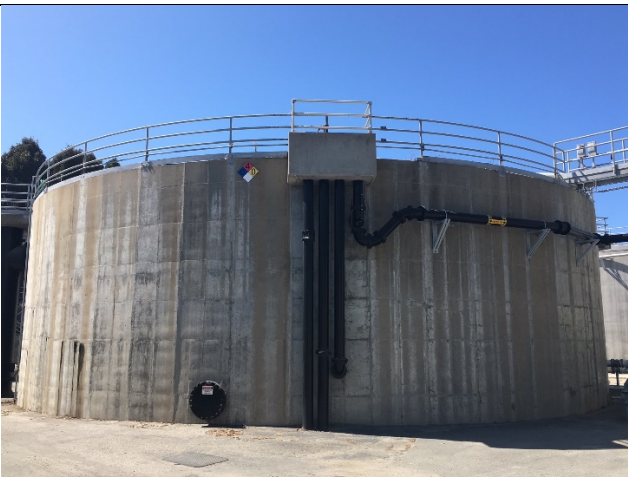
Photo: Digester No. 1
