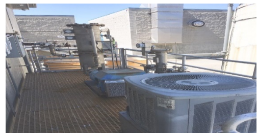
Photo: Existing Gas Conditioning System
