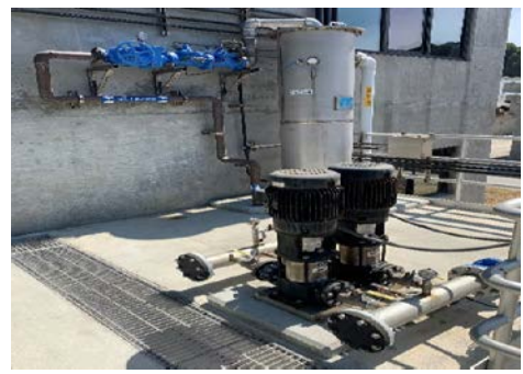
Photo: New #1 Water System where Corrosion System Project will be Installed
