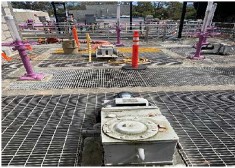
Photo: Existing Coagulation/Flocculation System and Sand Filters
