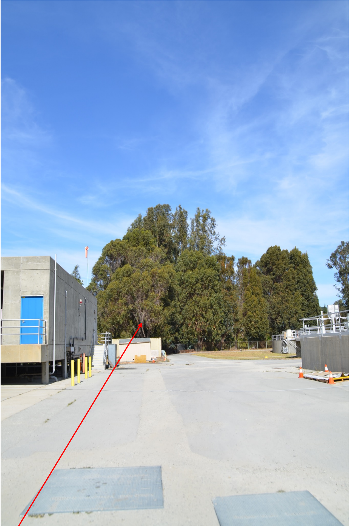
Tree next to storage tanks with fungal fruiting bodies observed at base.
