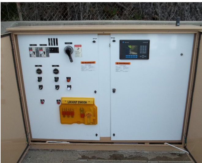
Photo: Pump station Control Panel- PLC and Operator Interface will be upgraded at Pump stations.
