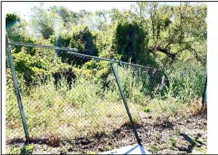
Photo: Existing Dilapidated Fence
