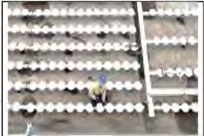
Photo: Existing air diffuser system
