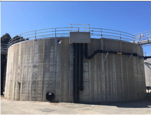
Photo: Digester No. 1
