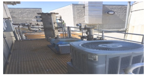
Photo: Existing Gas Conditioning System
