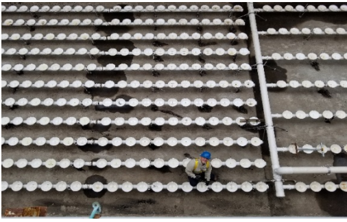
Photo: Existing air diffuser system
