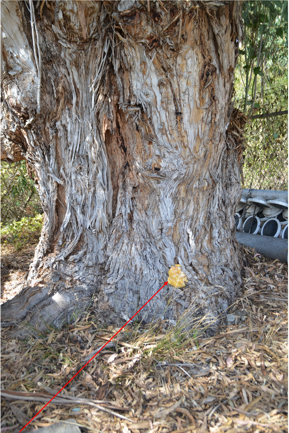
Fungal fruiting body on tree next to storage tanks in northwest corner.
