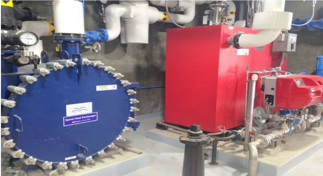
Digester Control Building #1 – Spiral Heater and Boiler
