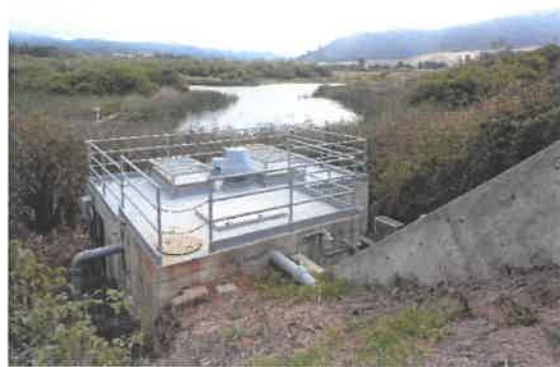
Calle la Cruz Pump Station
