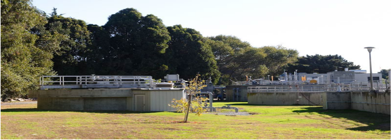
Clarifiers tanks & DAFT
