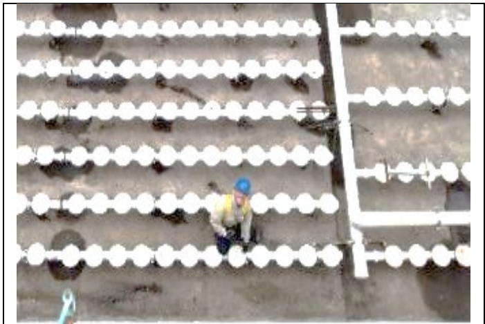
Photo: Existing air diffuser system
