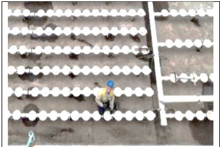
Photo: Existing air diffuser system
