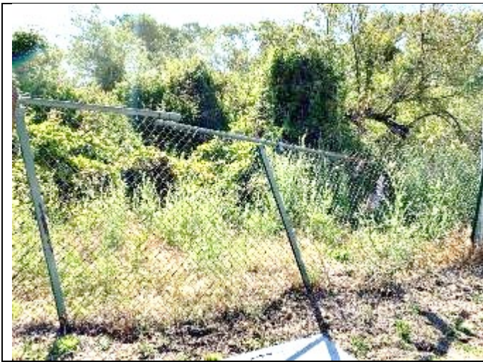
Photo: Existing dilapidated fence
