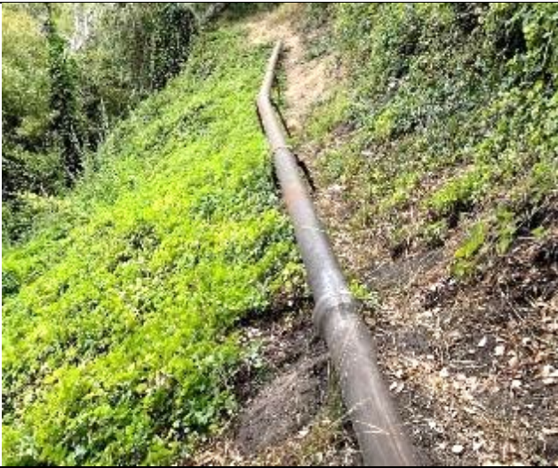
Photo: Sagged Pipeline
