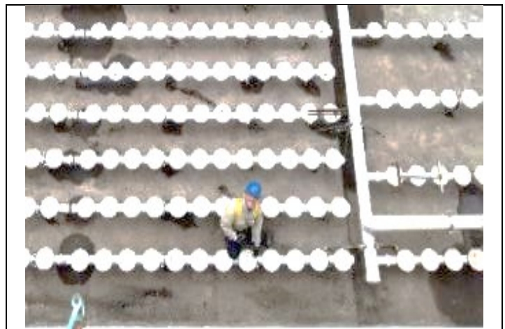
Photo: Existing air diffuser system
