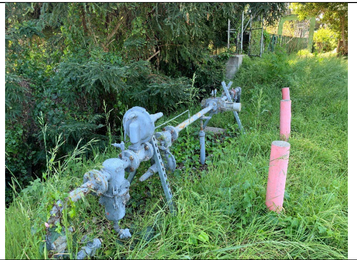
Photo: Gas Meter on North Side of River
