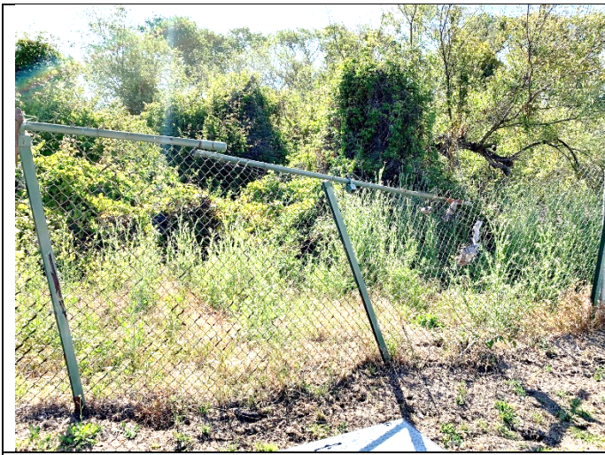
Photo: Existing Dilapidated Fence
