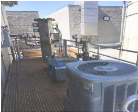
Photo: Existing Gas Conditioning System
