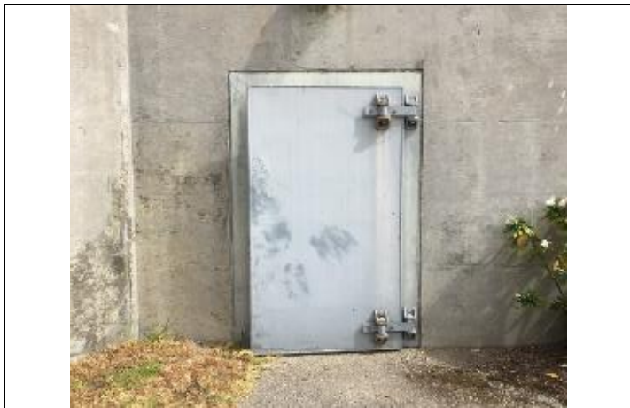
Photo: Old Flood Door in Headworks Basement
