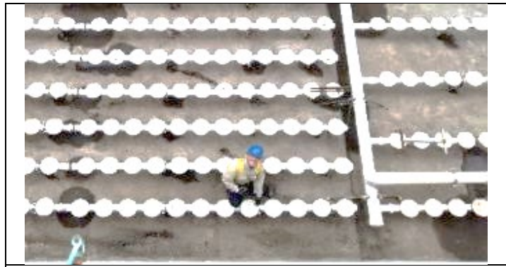
Photo: Existing air diffuser system
