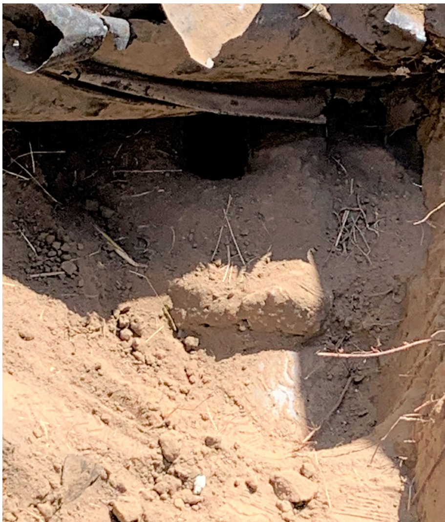
Photo No. 2- View of Water Line Above Existing Sewer and Hole In Sewer line
