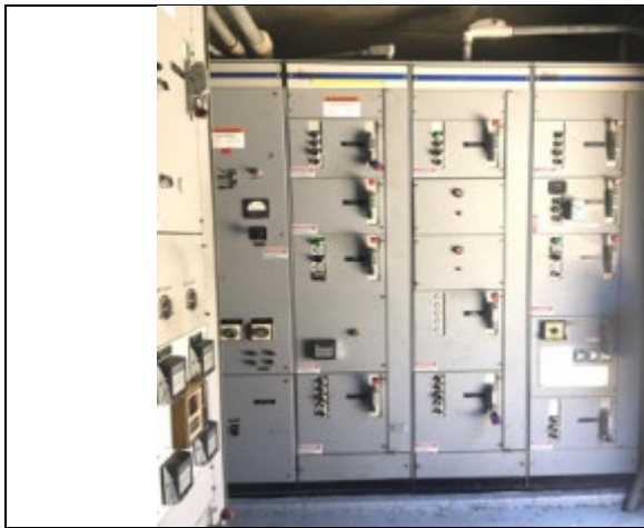
Photo: Existing Headworks Motor Control Center to Be Replaced in Project
