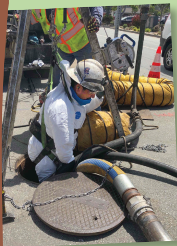
The Rio Road rehabilitation project protects our community’s investment by extending the useful life of the sewer line.
