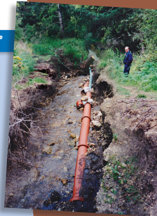
Hatton Creek has overspilled its banks during El Niño events, and high velocity flows have excavated CAWD mainlines. The Hatton Canyon Project will upgrade infrastructure to prevent spills and protect the environment.
