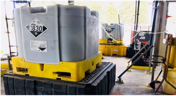
Photo: Existing totes used for Sulfuric Acid storage and Feed
