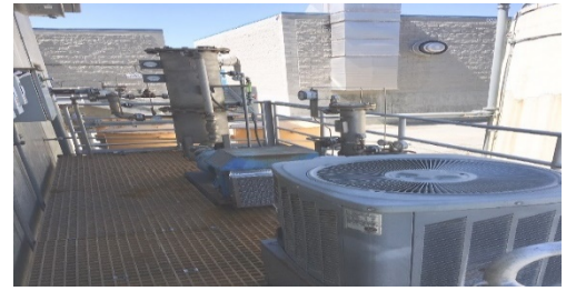
Photo: Existing Gas Conditioning System
