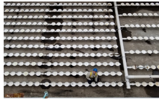
Photo: Existing air diffuser system
