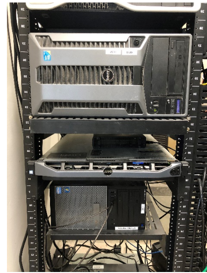
Photo: Existing Server Hardware that will be replaced in Project
