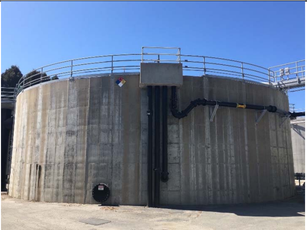
Photo: Digester No. 1
