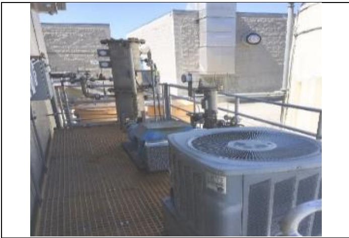
Photo: Existing Gas Conditioning System
