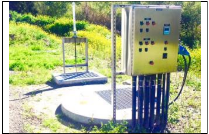
Photo: WWTP Stormwater Pump Station
