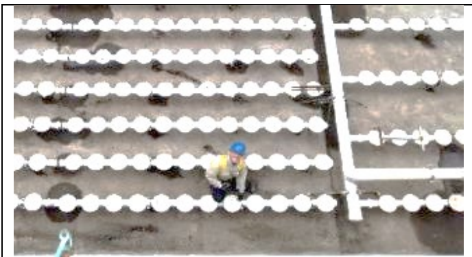
Photo: Existing air diffuser system
