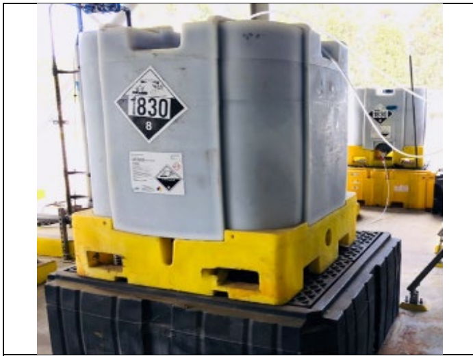
Photo: Existing totes used for Sulfuric Acid storage and Feed
