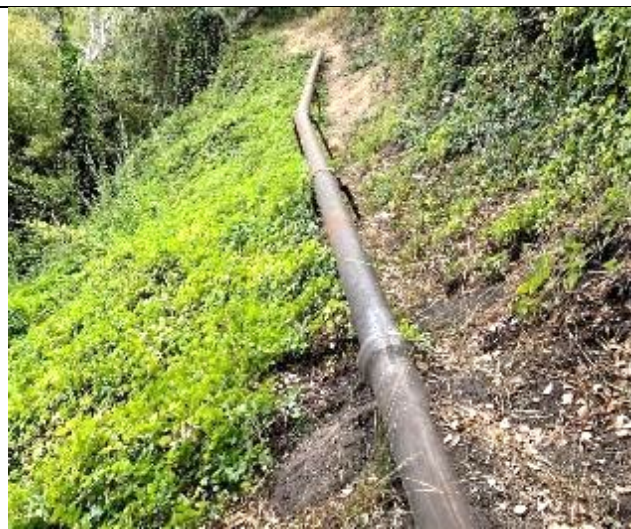
Photo: Sagged Pipeline
